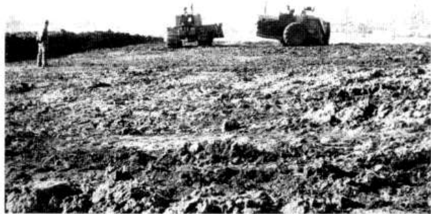
EARTH-MOVING machines claw into the ground to prepare the site for the new Westport Road High School.
